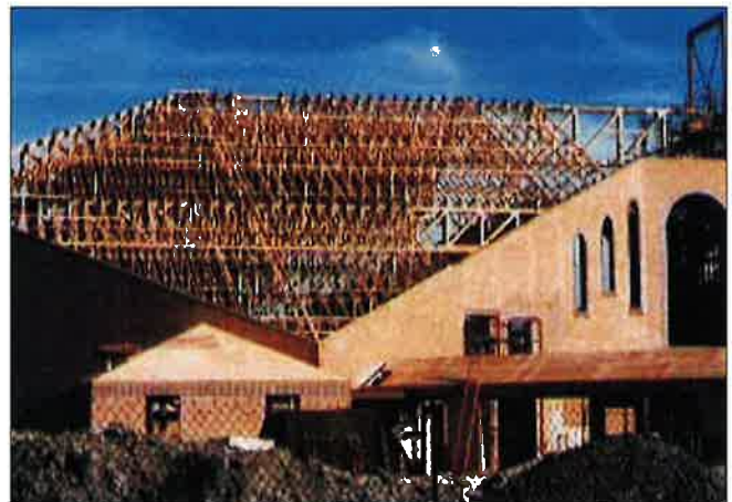
In addition to residential component products, CCC specializes in commercial and multi-family projects. For example, this church was constructed for the St. Lucy’s Parish in Racine. Its 6/12 roofpitch spans 174 feet and incorporates 115 truss designs. The roof is supported by three girders. The main girder is nearly 91 feet long and all are 10 ply. WTCA featured this project at the National Association of Home Builders show in 1997.
